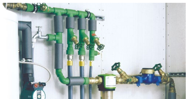
House connection station
